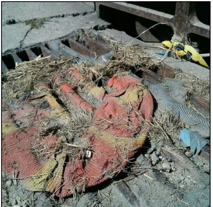
...and not neglect the drain protections.
